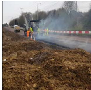
Work started on Phase 3 of the improvement works on A350 Chippenham Bypass.
