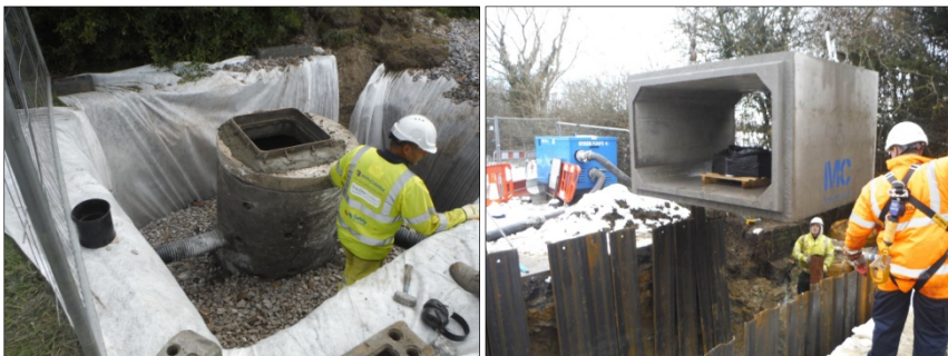
The Council has carried out drainage improvement and flood alleviation schemes across the county.
