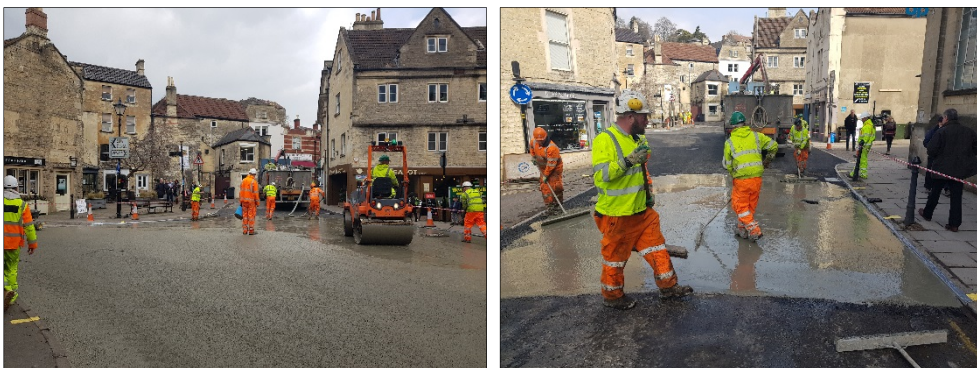
Grouted Asphalt was used at Bradford on Avon to provide a durable road surface.
